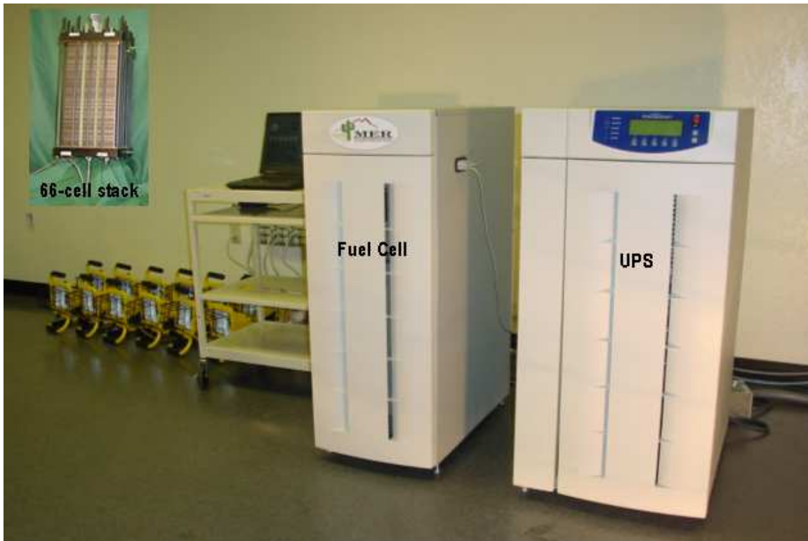
Fig.1: MER's 13 kW Fuel Cell UPS system.
